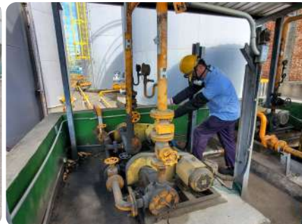
Close the raw material gate valve
